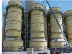
Owners of coal-fired power plants invested more than $30 billion in flue gas desulfurization systems , also known as scrubbers, between 2007 and 2011, according to a report from the U.S. Energy Information Administration.
